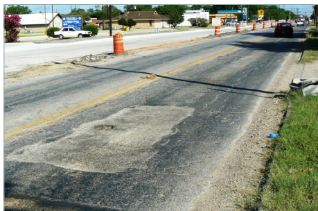
Typical 6" deteriorating asphalt arterial in Victoria
